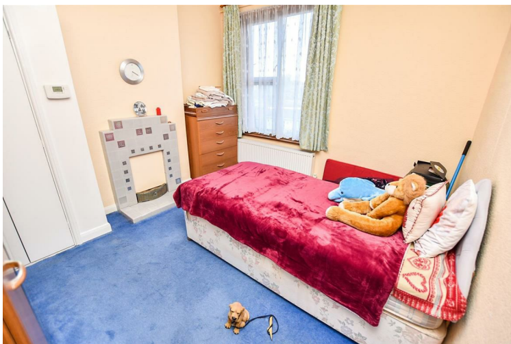
Window to rear, radiator, cupboard housing Vaillant gas combi boiler,
